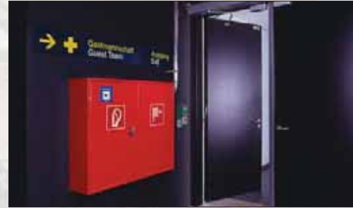
Fire and smoke protection doors
